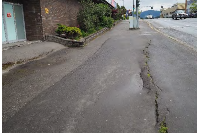
Uneven and cracked sidewalk on 2 nd Avenue West
