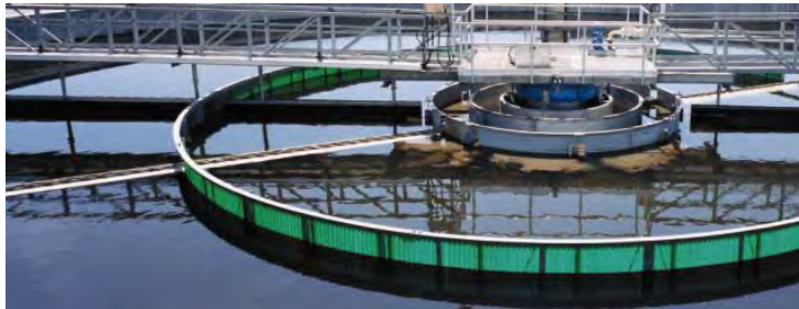
Figure 4-1 Existing Primary Clarifier
