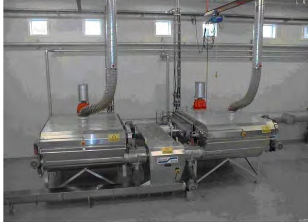
Figure 4-5 Existing Micro Screen Installation
