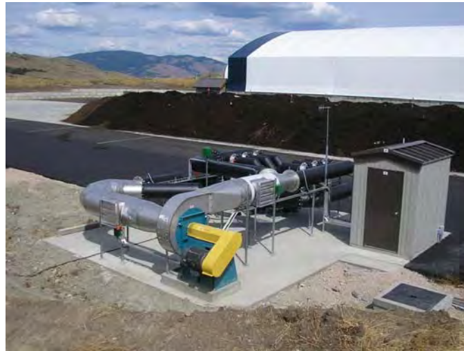
Figure 4-1 Kelowna/Vernon Composting Facility (Source: Engineered Compost Systems , 2007)
