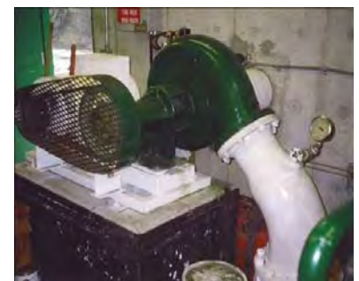
A typical small-scale PAT installation. Source: Associated Engineering
